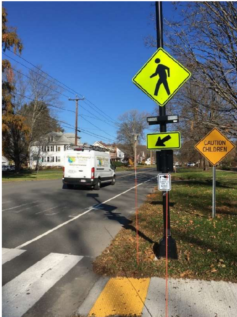
Hatfield DPW installed Rectangular Rapid Flashing Beacons pedestrian actuated signals on the Main Street intersection with North Street in 2023 as an effective safety initiative.
